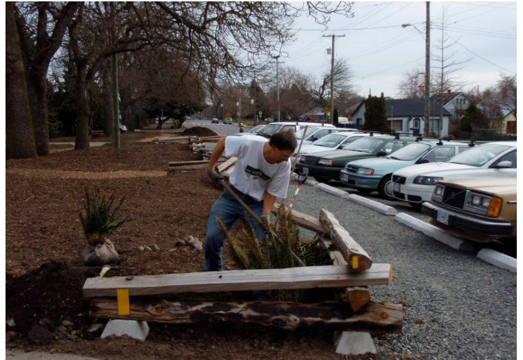
Wooden fence installation (Note concrete wheel stops in front of cars on the right)
